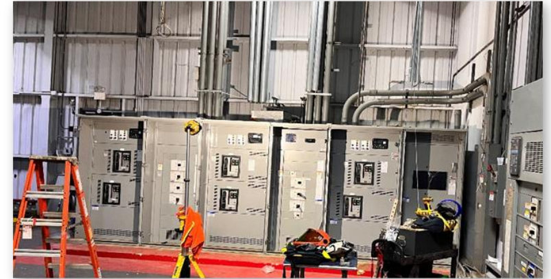
Replaced Eaton's aging switchgear with intelligent power distribution equipment that has paralleling capability
