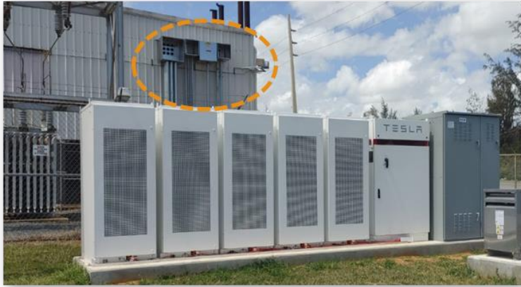
Installed new conduits to route power sources to the centralized switchgear and controls
